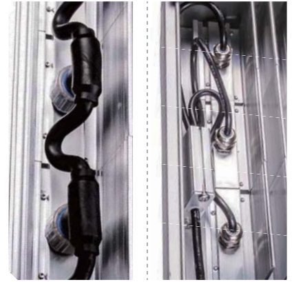
New connection, neat, clean and efficiency
